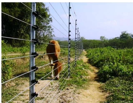
Solar Power Fencing
