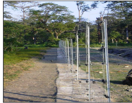
Solar Power Fencing
