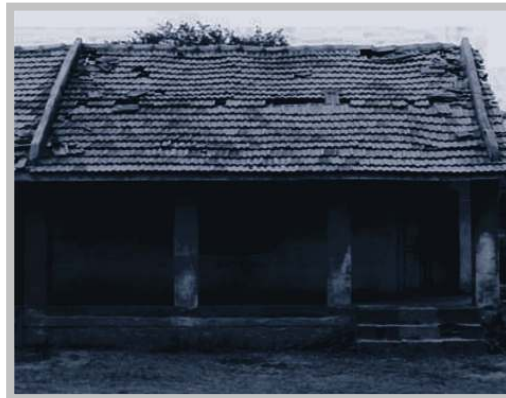
Damaged roof of Salagame School building, Hassan Taluk.
