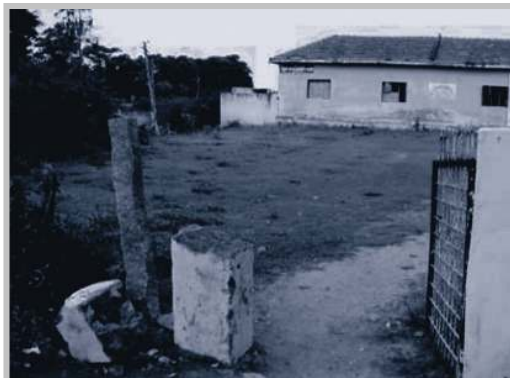
Broken gate and fencing in Salagame School, Hassan Taluk.
