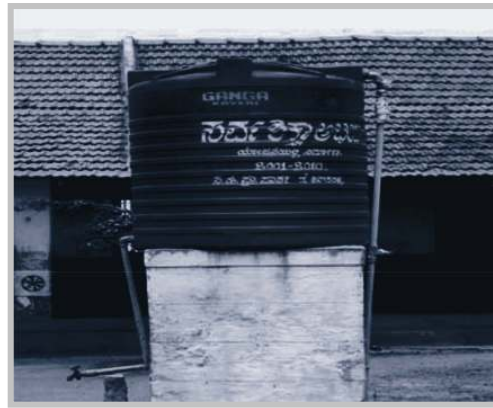
Water tank constructed under SSA fund left unused, as there is no water supply, Anugavalli School, Hassan Taluk.
