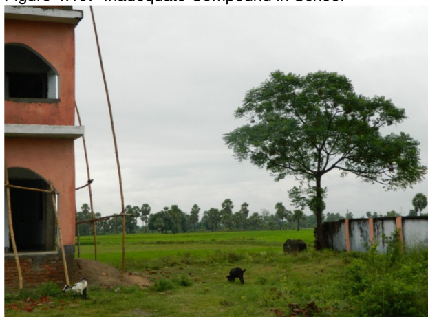
Figure 4.19: Inadequate Compound in School
