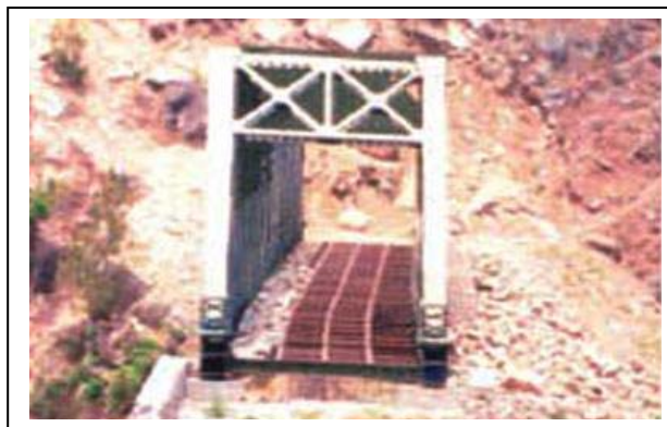
Incomplete and defective bridge over Tonse River
