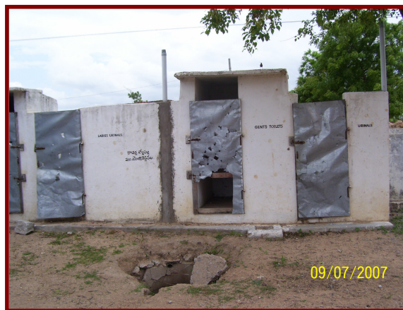
Toilet Blocks in schools have unhygienic conditions and are not properly maintained
