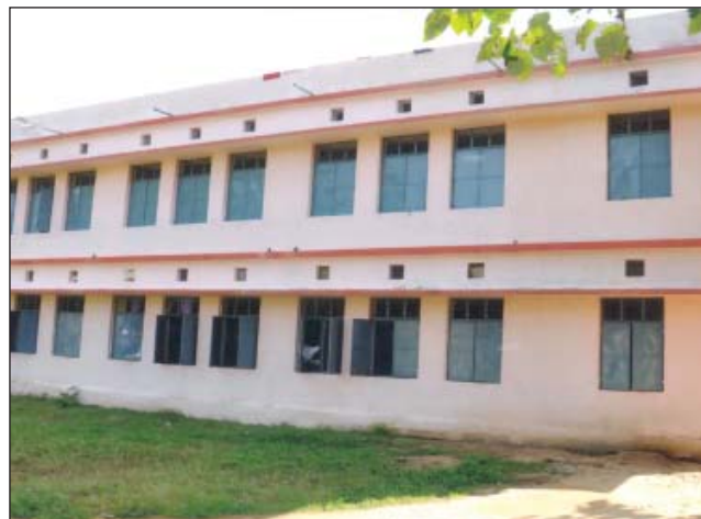
Constn. of 1 st . floor hostel building for Boys hostel at Bhalulata H/S under Bisra block
