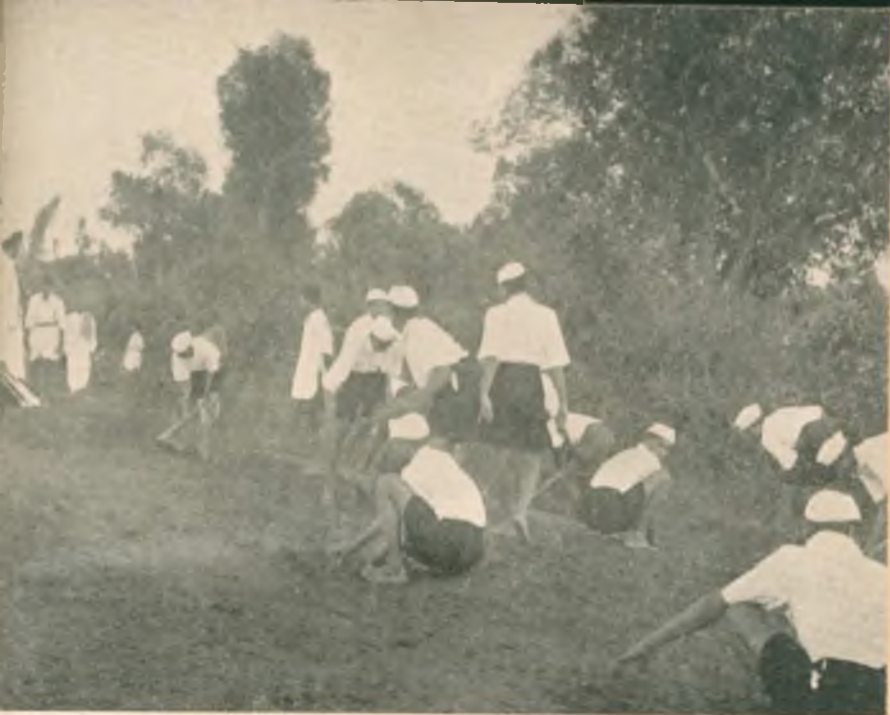
Seva Dal workers building a road in the village of Thadagani in Mysore.
