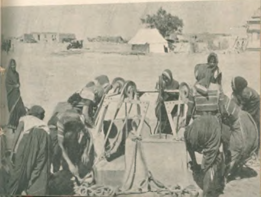
This well is one of the many constructed in Hyderabad community project area.
