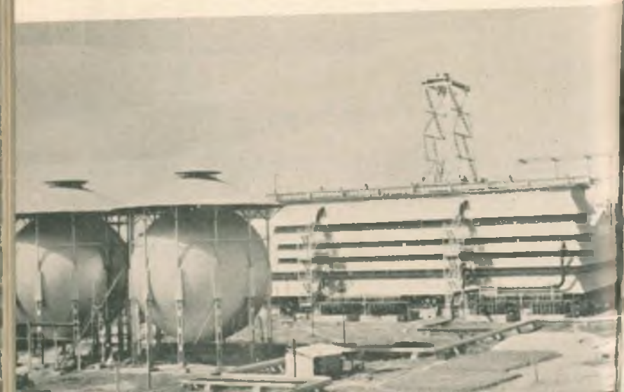
A view of the ammonia synthesis plant of the Sindri Fertilizer Factory.
