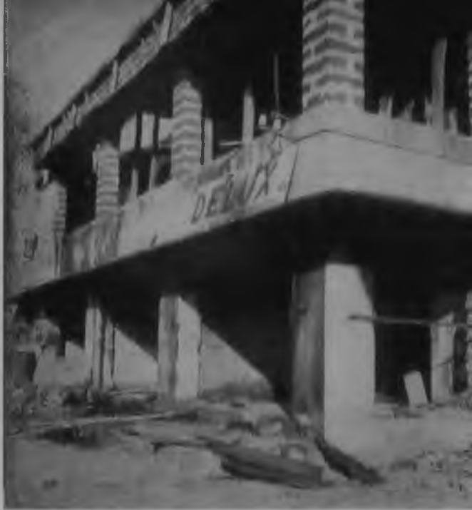
A scene showing a portion of the burnt and damaged building of Shri Satyapriya Mohanty
