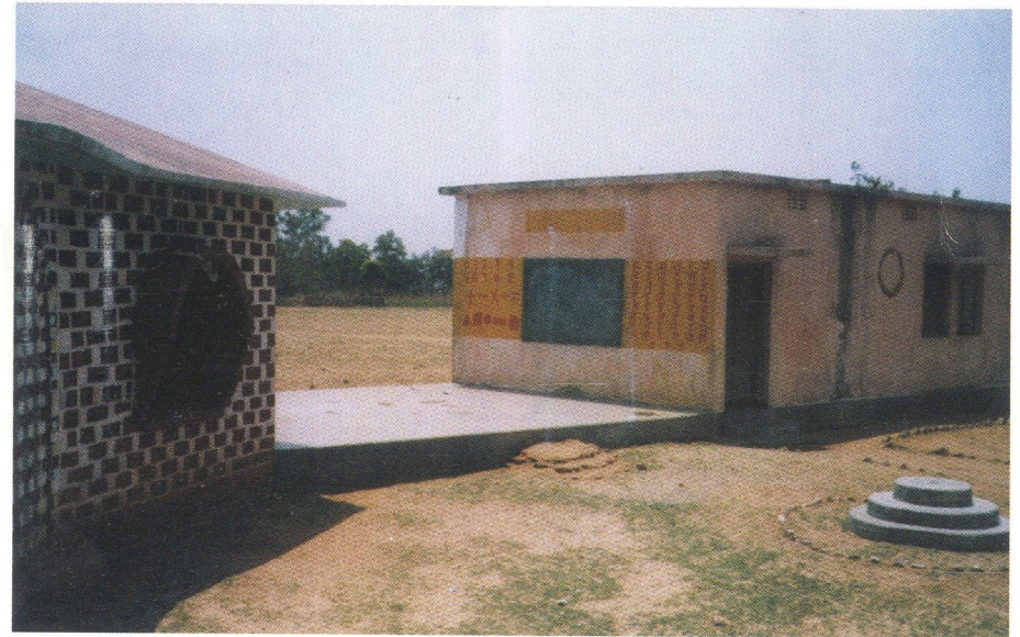
*** A platform provided between two existing classrooms. The chalkboard is placed on an existing wall. In future, this platform can be easily built upon, and two walls will be saved.
