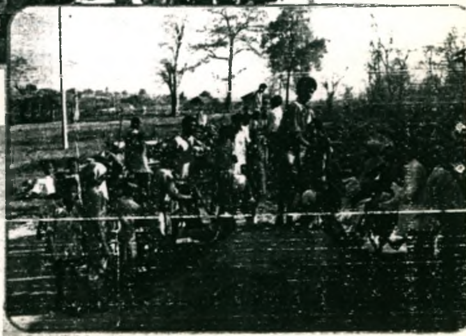
VEC members on work for the school building at Devadumula village Eturunagaram Mandal Warangal Dt.
