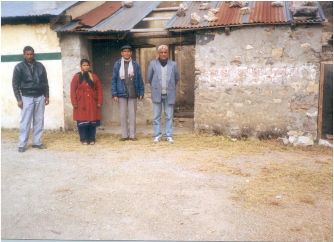
Roofless building of Primary School Dakra (Photo 2)
