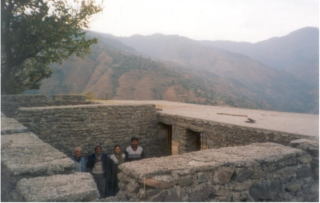
Roofless building of Primary School Duniyara (Photo 1)
