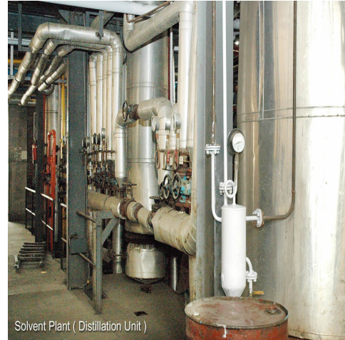
Solvent Plant ( Distillation Unit )
