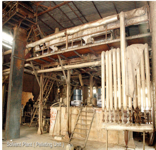
Solvent Plant ( Pelleting Unit )
