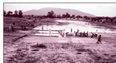
2.5.17 Work in progress at Chhatna where both men & women SHGs are working together (a RSVY project)
