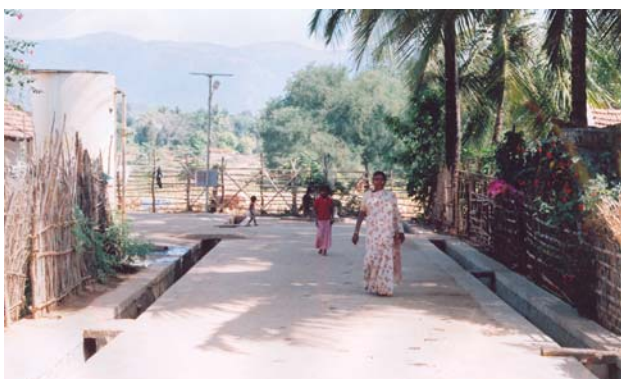
Road and drainage, mini water supply, solar street light provided under Article 275(1) of the Constitution of India grants at Banawadi scheduled tribe cluster in Chamarajanagara district of Karnataka
