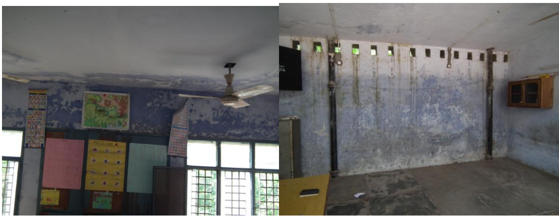
SEAPAGE IN SCHOOL BUILDING- CLASSROOMS OF GMHS SECTOR-12 & GPS- SECTOR-12
