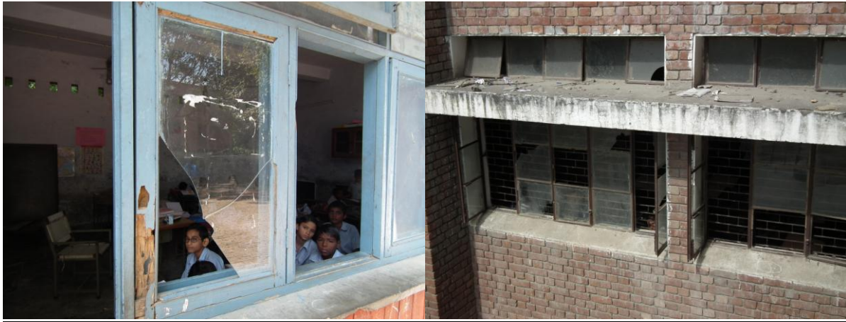
BROKEN WINDOW PANES OF CLASSROOMS OF GPS-12 & GMS-52
