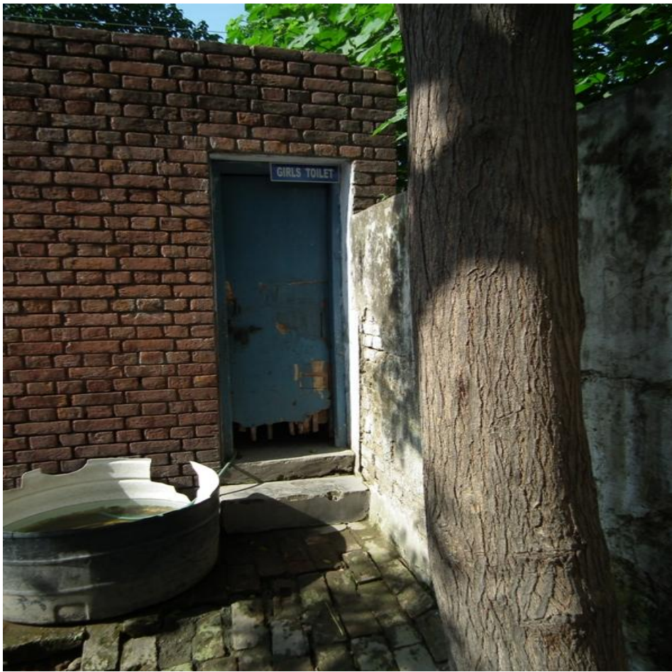
BROKEN DOOR OF GPS- SECTOR-12 GIRLS TOILET
