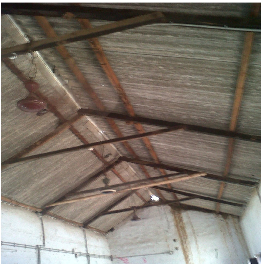
(Leaking temporary roof in a DIET classroom)
