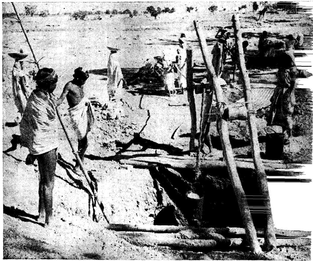
With a cent per cent Government subsidy this well is being dug up in an Adivasi village of Ranchi.
