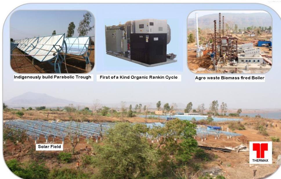
Figure 3. Decentralized solar energy Plant in Shive, Maharashtra
