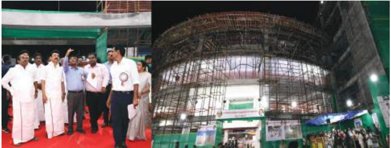
The Hon'ble Chief Minister of Tamil Nadu Thiru.M.K.Stalin inspected the progress of construction work of the Kalaingar Centenary Library at Madurai on 07.06.2022.
