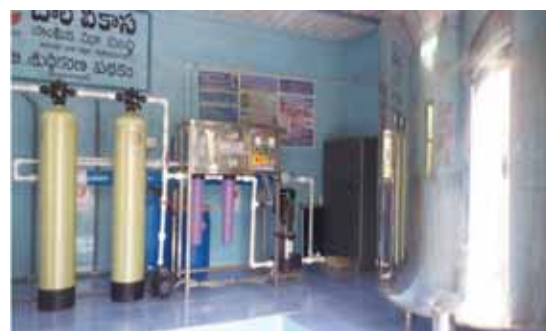
Solar street lights Water purification plants
