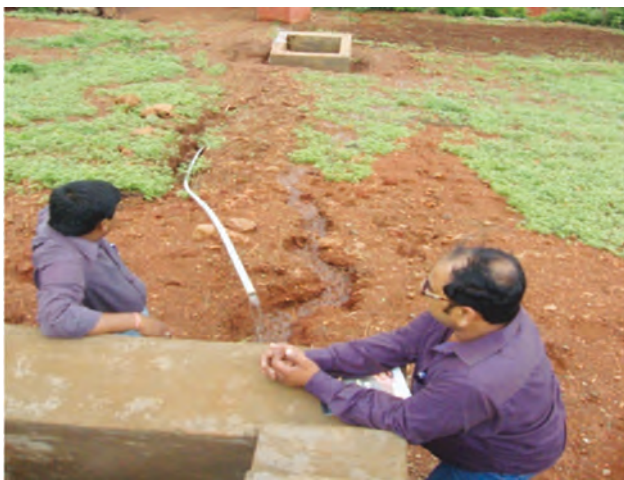
Ongoing hydram project lifting water to uphill for irrigation
