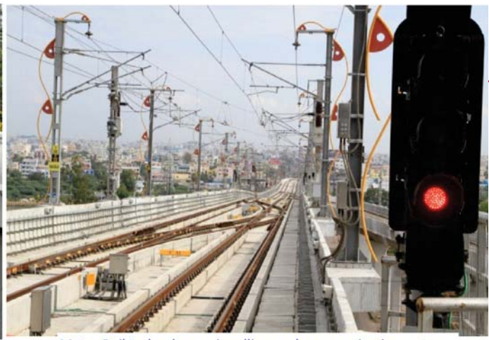
Metro Rail technology –signalling and communication system
