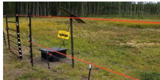
Solar Powered Battery Fencing
