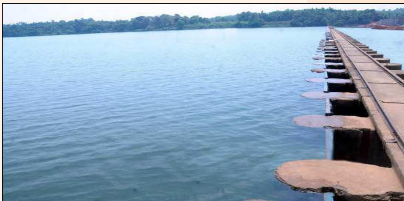
Vented Dam at Thumbe - A source of water supply to the Mangaluru city
