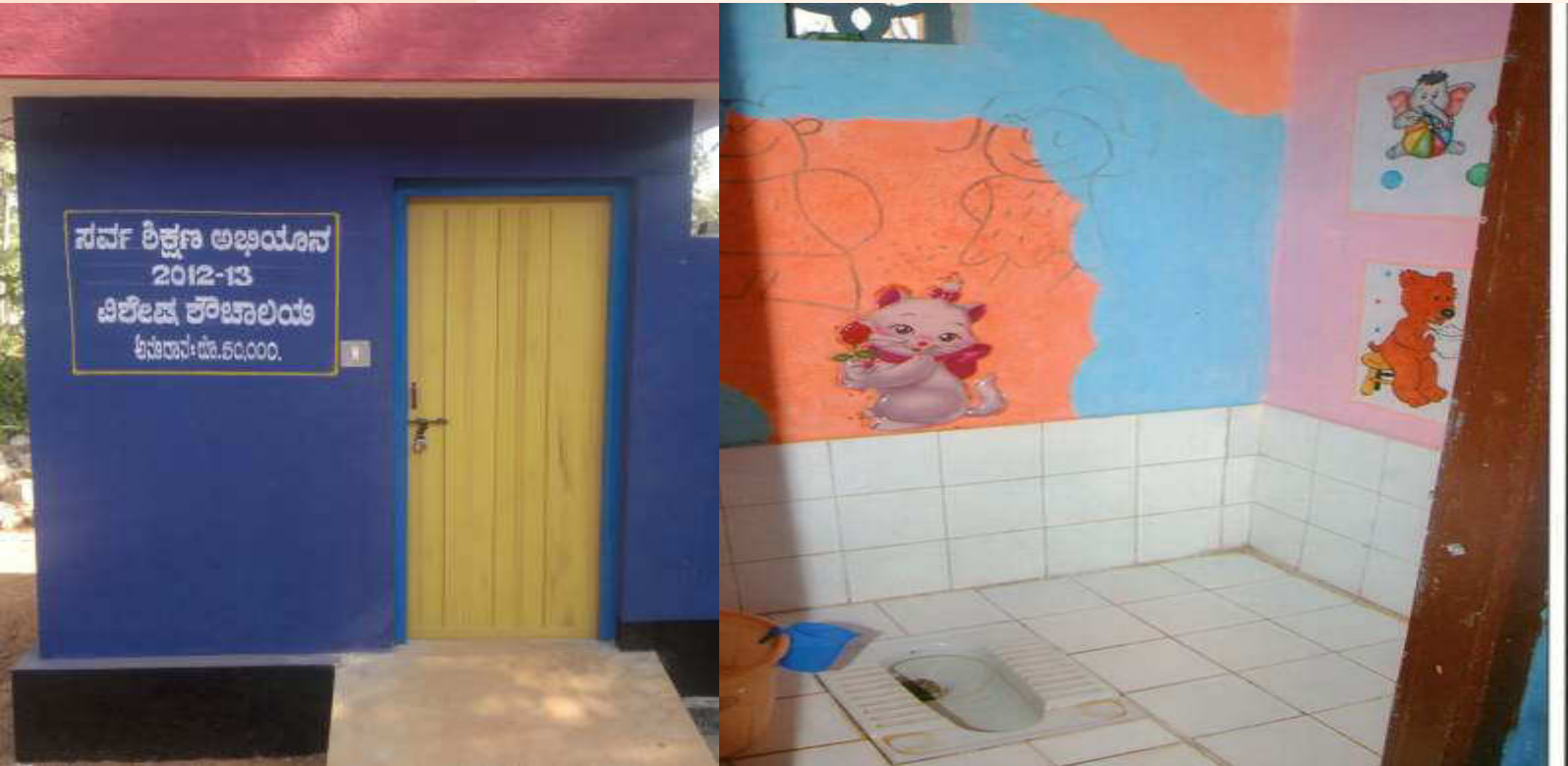
Toilets Designed Exclusively for Anganavadi Children
