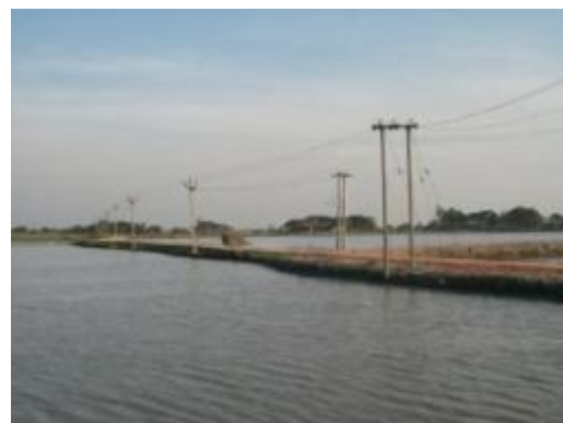
ELECTRICITY CONNECTION TO TENTULIA VILLAGE, WEST BENGAL
