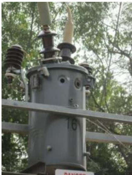
THEFT OF 'COPPER WOUND' FROM THIS TRANSFORMER
