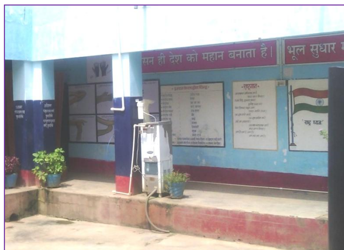
Water facility for MDM
