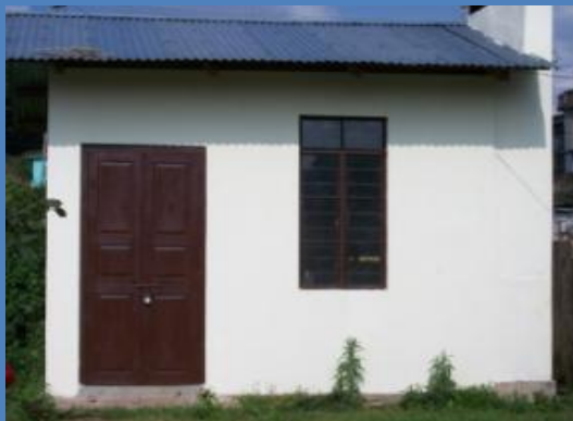
Constructed kitchen shed for Mother Union Ampati Upper Primary school of Betasingh block of West Garo Hills District.
