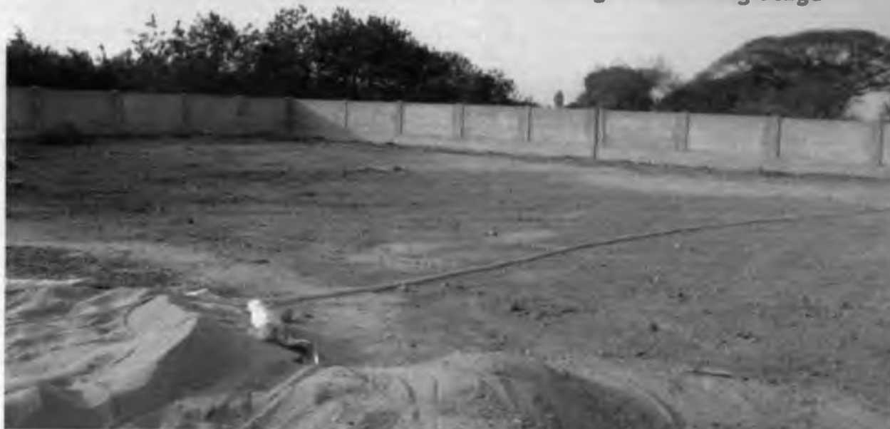
N/w : Construction of Shandy (Village Hatt) at Morampally Banjara of Burgampahad (M) in Khammam District. (Compound wall) Esst. Cost : 7.00 Lakhs Grant : IAP(LWE) Sector : Livelyhood Activities Stage : Finishing Stage
