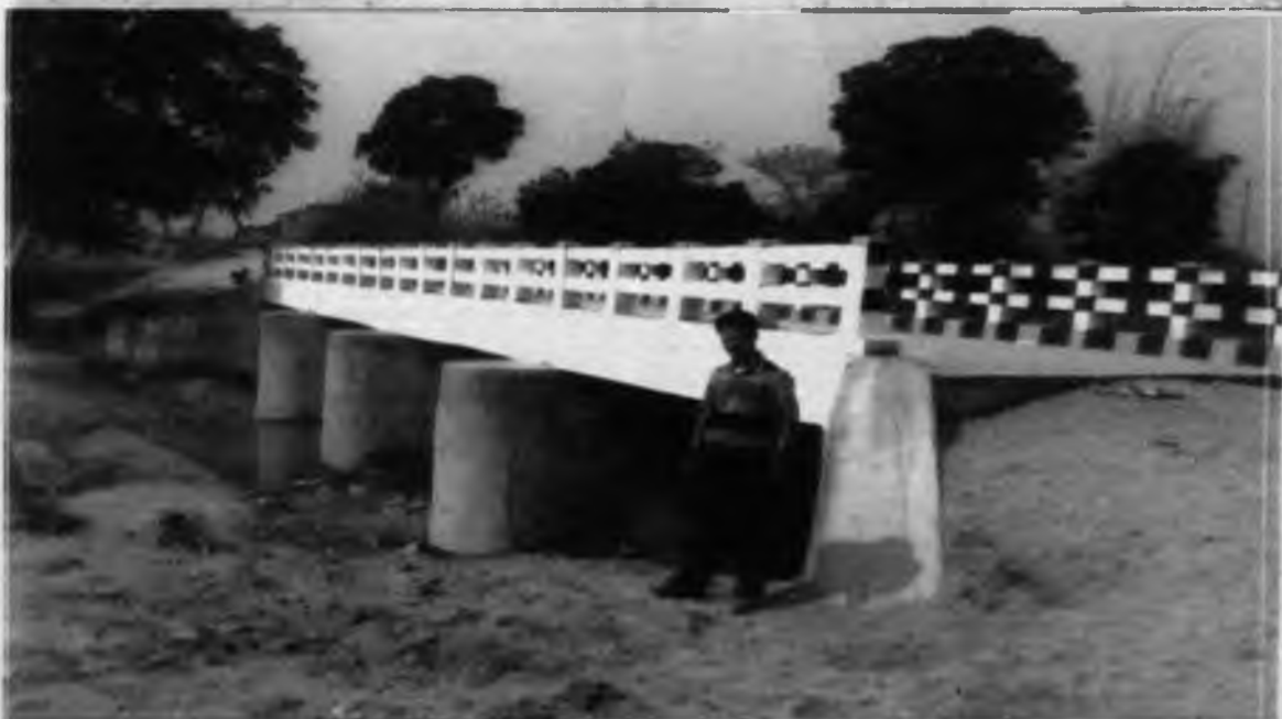
Typical four span Bridge constructed under IAP. This is a four span Bridge constructed over Sira nala in village Nawadih in Chatra Block.
