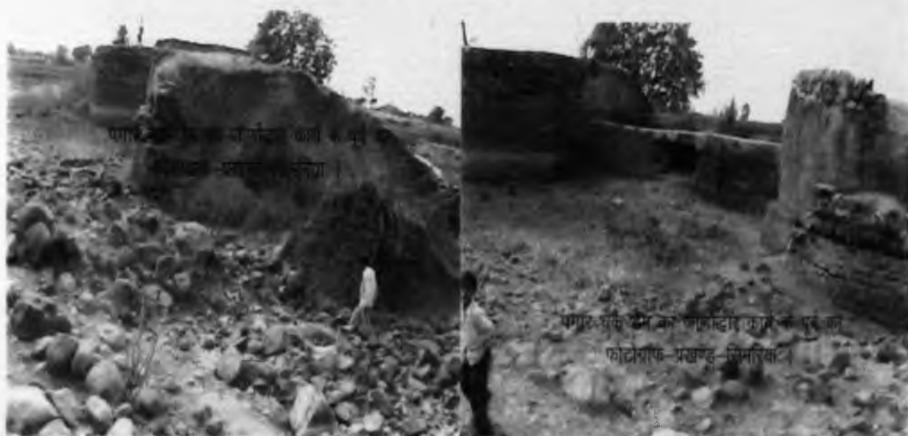
Breach in the pagar dam and old check dam in dilapidated condition
