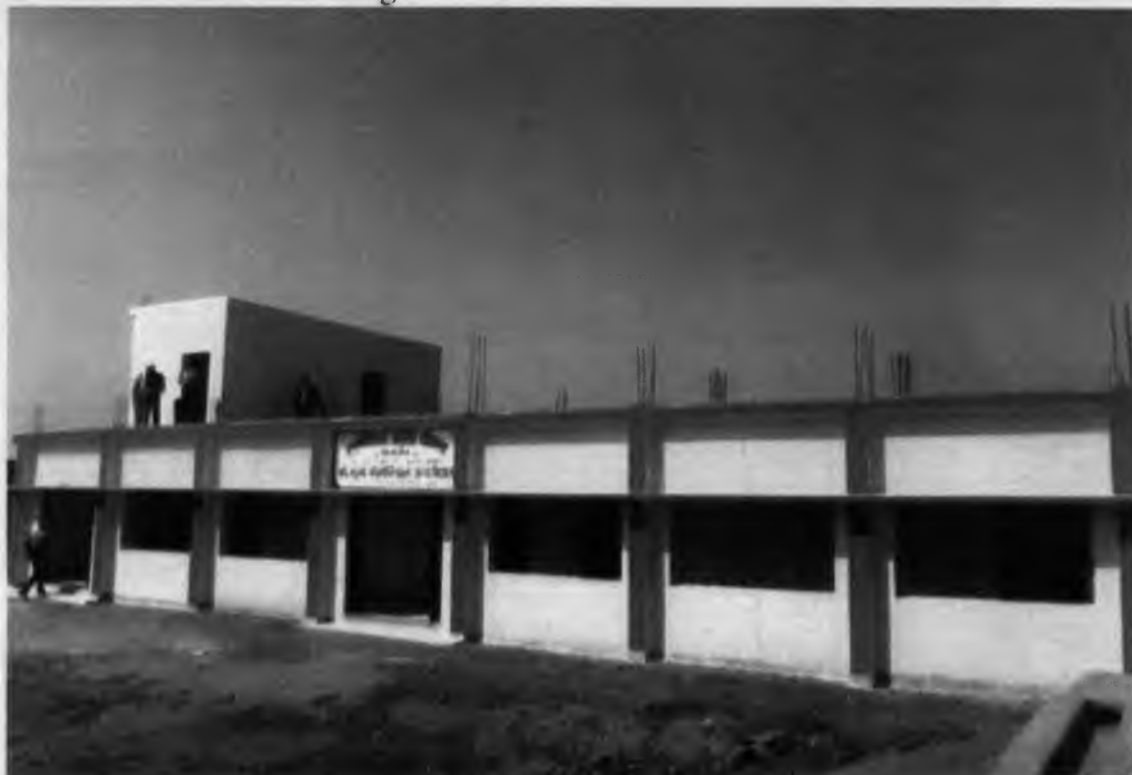
Typical two addition classroom building provided to educational institution under IAP .This photo is of Musa Memorial High School, Chatra.
