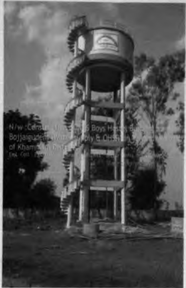
N/w :Construction of AHS Girls Hostel Building at Rampadu, Water supply & OHS in Yellandu Mandal of Khammam District. Est. Cost : 25.00 Lakhs. Gram : JAPILWE. Sector : Intro. to DCC, MMS, etc. Stage : Completed
