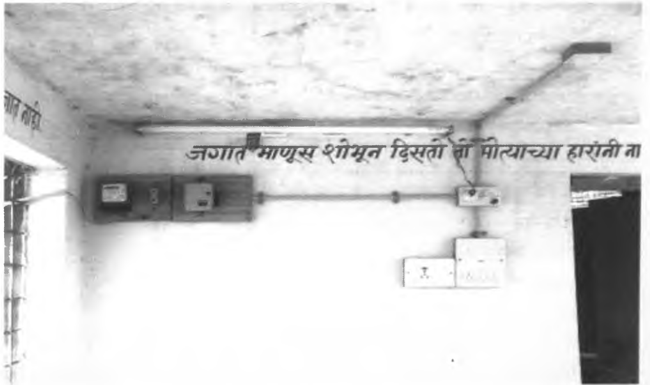
School Electrification- Z.P.School, Darbha, Tah.Bhamaragad
