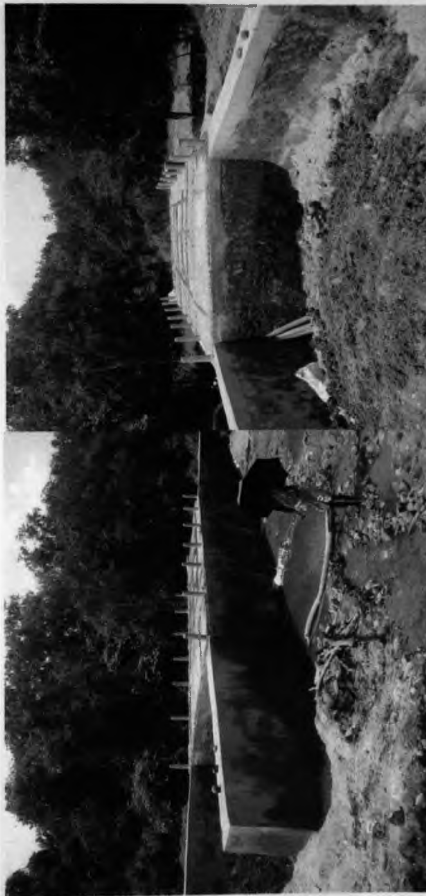
Construction of CD work from Jashipur to Ghutudihi road Barei Nallah in Jashipur G.P., Bahalda Block. Rs. 14.00 Lakhs. This is benefitting 200 families (approx)
